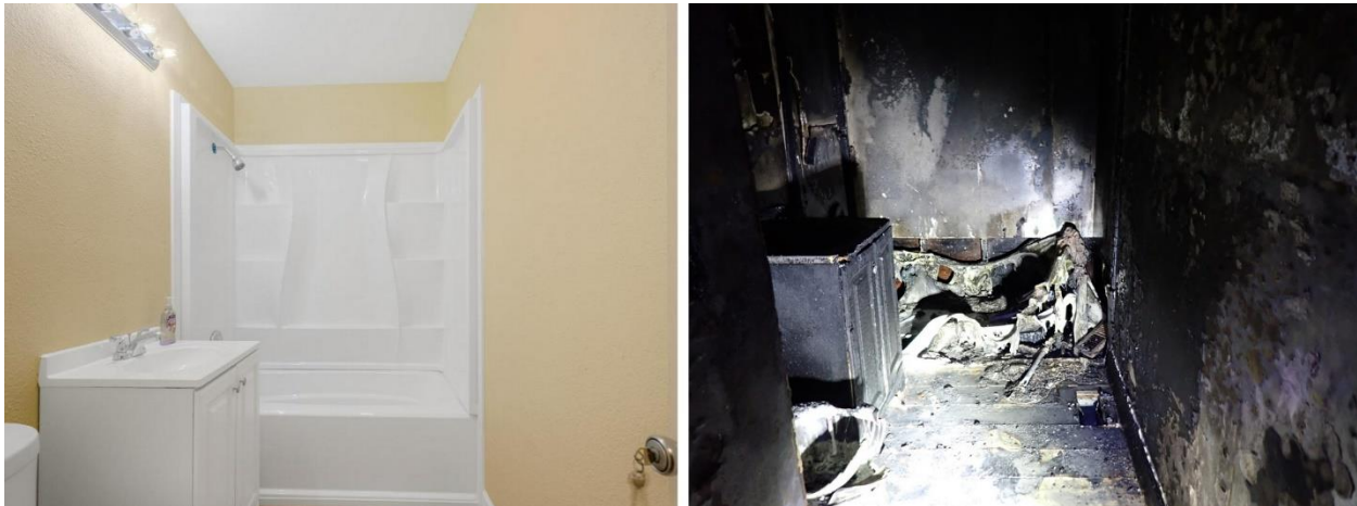
Figure 25. Pre- and Post-Fire Photos of the Bathroom
