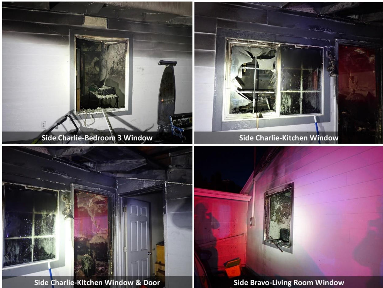
Figure 46. Ventilation Openings on Sides Charlie and Bravo
