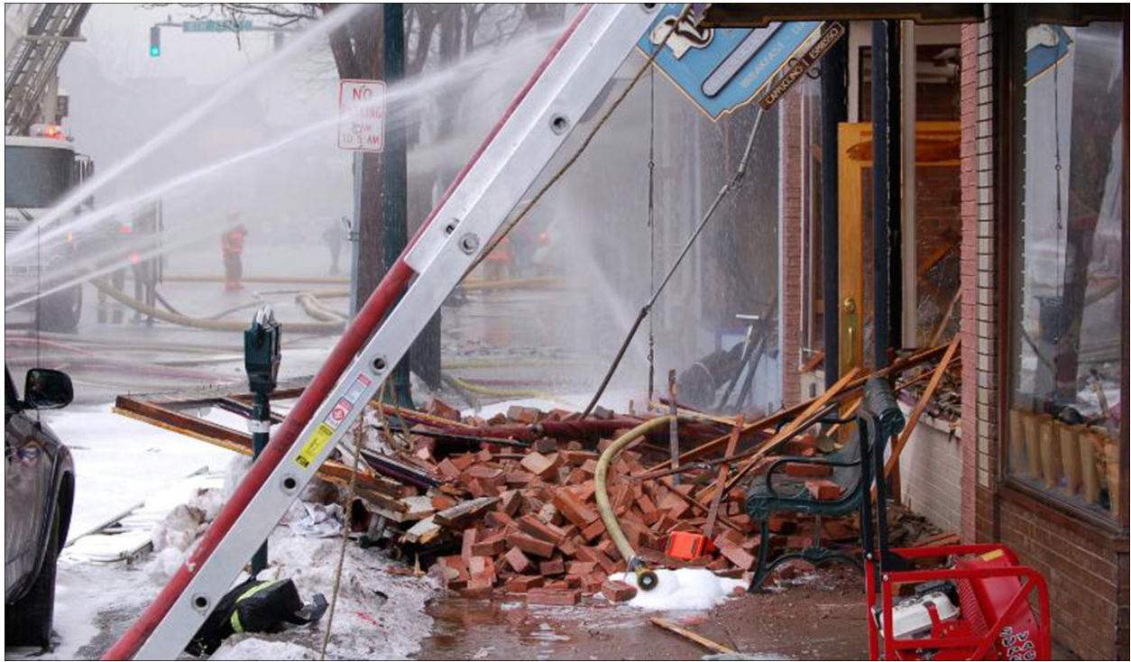
Figure 14. Looking North (towards Side B) on Side A In Front of Exposure D2.
