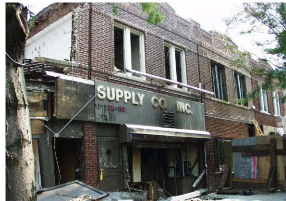
Figure 1. Side Alpha-Post Fire
