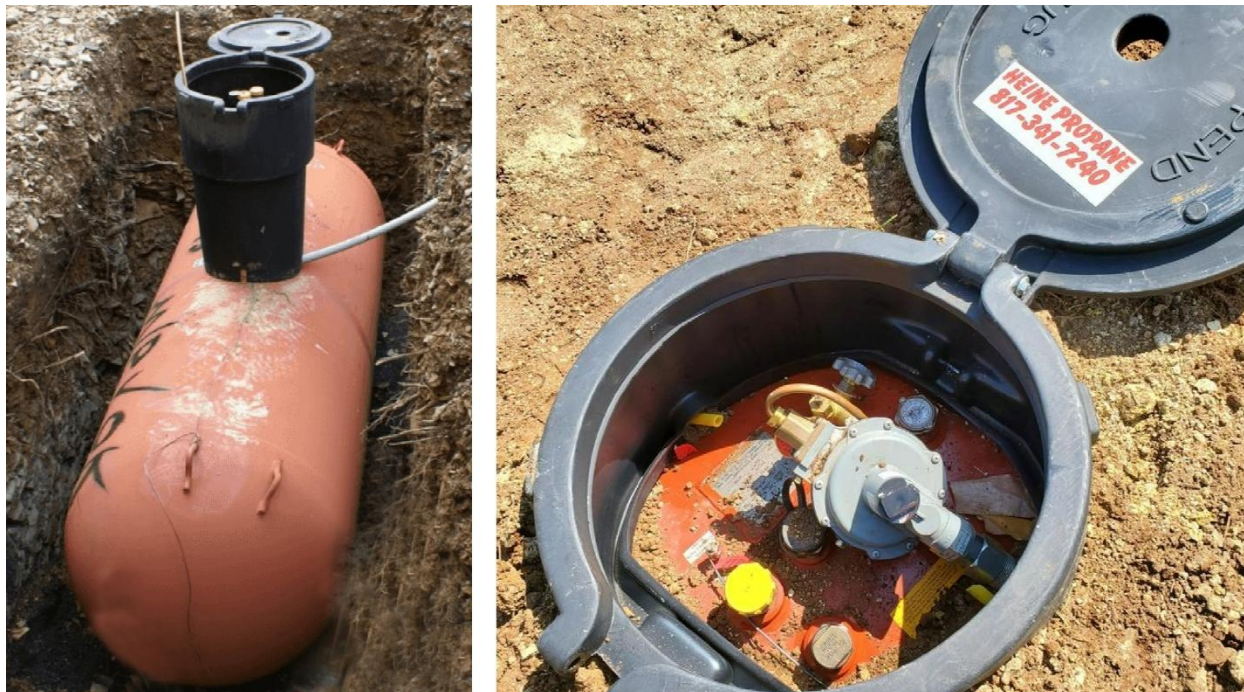
Figure 11. Similar Underground Propane Tank Installation
