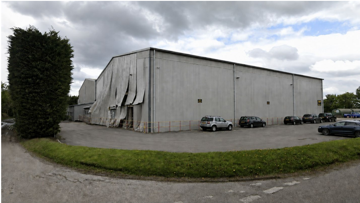
Figure 6. Conditions on Side Charlie (View from the Bravo/Charlie Corner)
